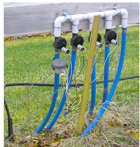
FIGURE 16. Valve bank with an automated controller in a vineyard.
